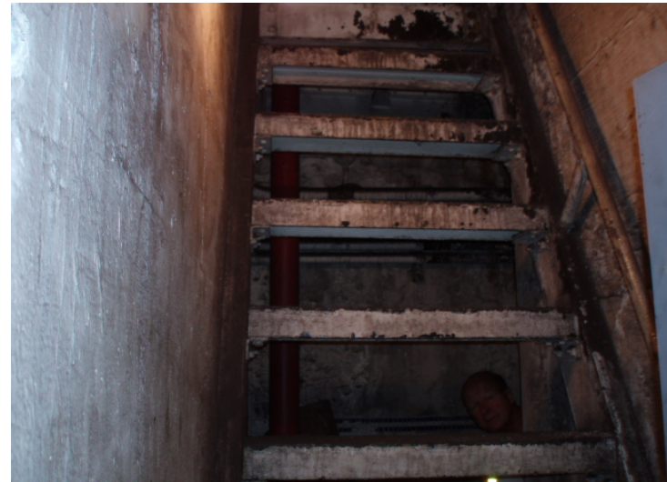
6. View of a steel stairwell and railing located at an emergency exit within Bowdoin Street Station. The stairwell is coated in paint suspected to be lead-based.
