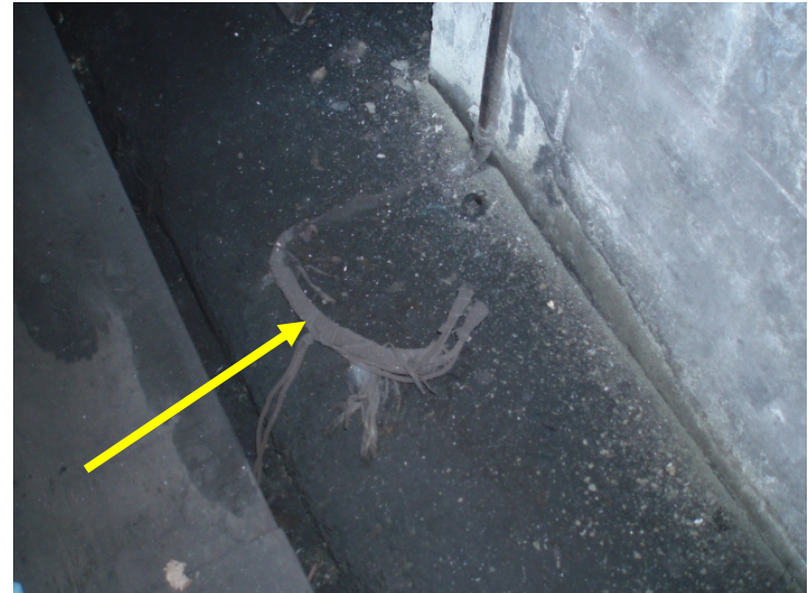
16. View of suspect asbestos-containing, woven wire insulation found in Bowdoin Yard Tunnel
