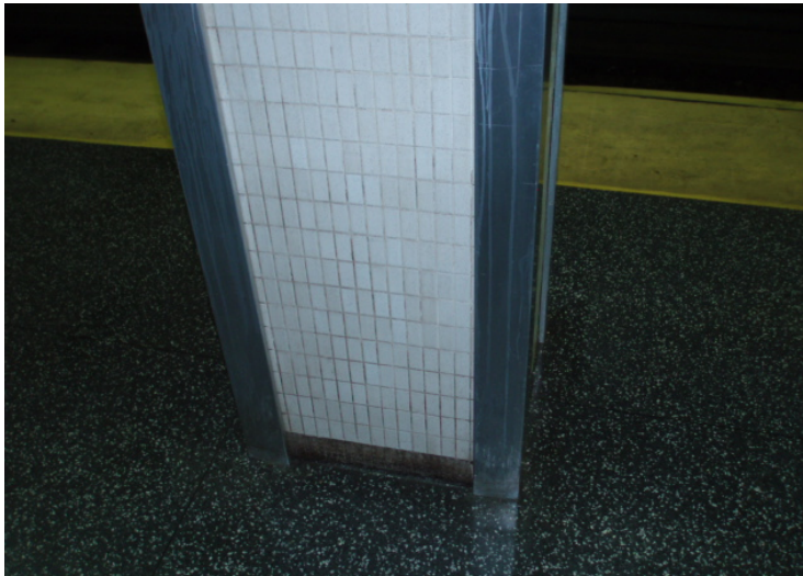
5. View of white ceramic tiles suspected to contain lead. The tiles were observed on support columns and walls in various areas throughout the Project Corridor.
