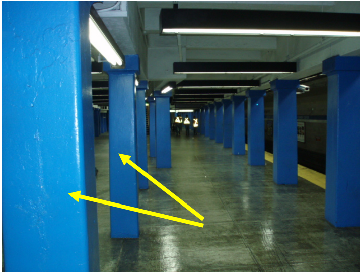
11. View of painted support columns suspected to contain lead-based paint.
