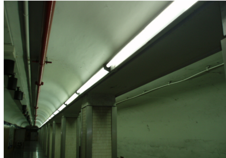
2. View of fluorescent light fixtures observed in various lighted areas throughout the Project Corridor. The fixtures contain suspect PCB-containing ballasts.
