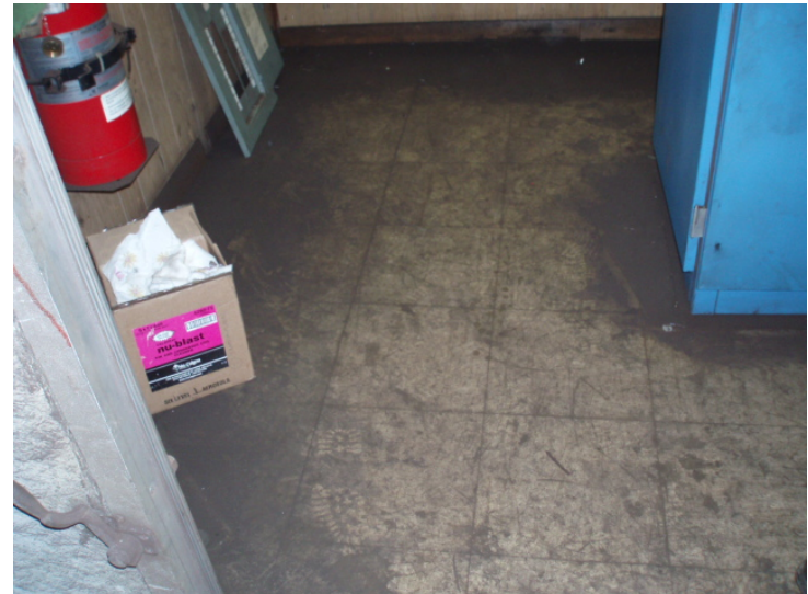
14. View of suspect asbestos-containing vinyl floor tiles located within a communications room within the Project Corridor.
