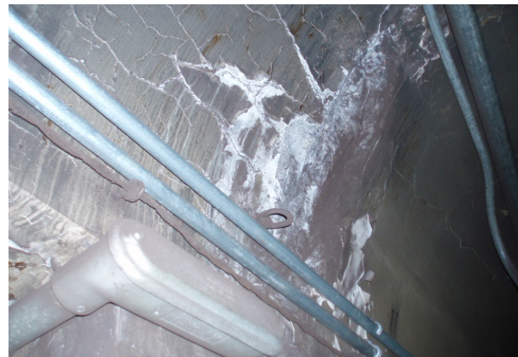
4. View of damaged suspect asbestos-containing plaster skim coat. The painted surface of the skim coat is suspected to contain lead-based paint.
