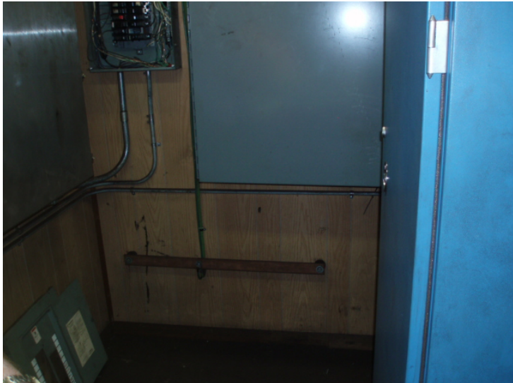
15. View of wood wall paneling and suspect asbestos-containing wall panel glue located within a communications room.
