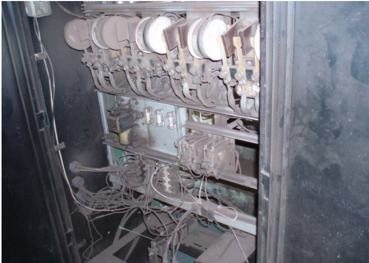
1. View of suspect asbestos-containing transite discs located in an electrical room within Bowdoin Street Station.
