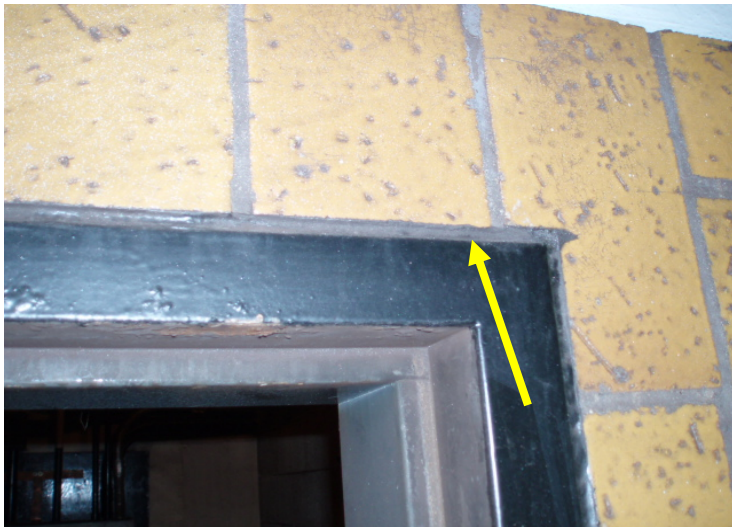
7. View of suspect PCB/asbestos-containing caulking typically found around door frames within the Project Corridor.
